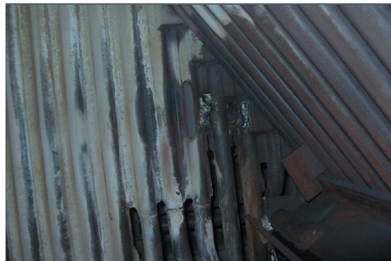
Figure 10: An example of typical boiler tube failure locations
